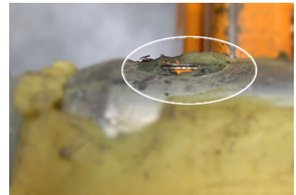
Protruding Shear Bolt
